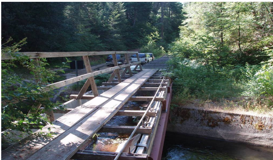
Figure 5. The existing Esmeralda Creek diversion. July 2007.
