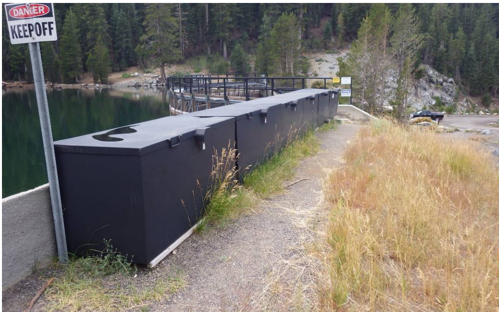
Photo B4 – Stop Log Storage Bins
