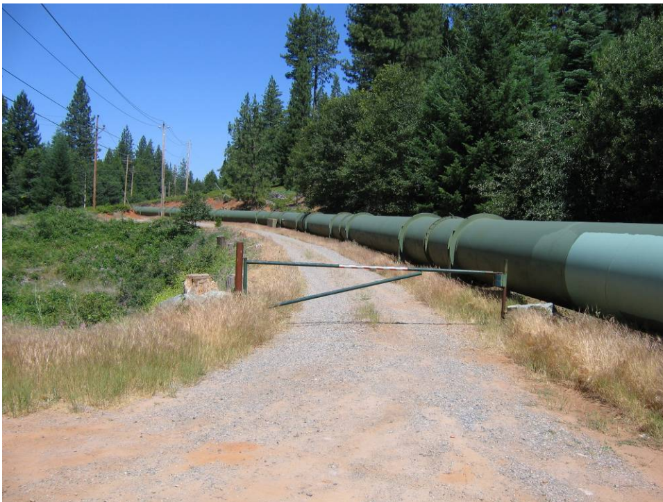
Photograph B-30. El Dorado Pipeline.
