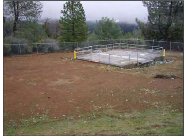
Photo 8 – Existing Pressure Reducing Station at Reservoir B
