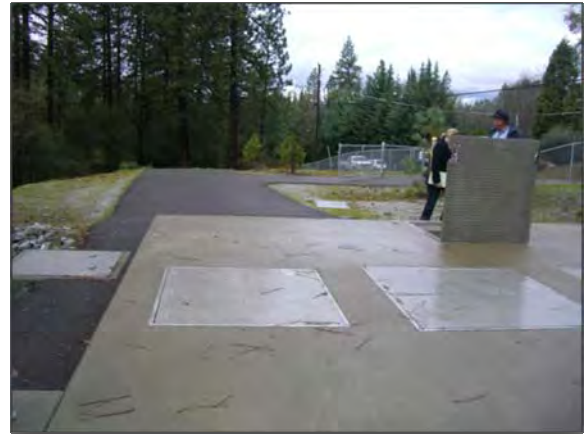
Photo 10 – DSM Pressure Reducing Station No.1
