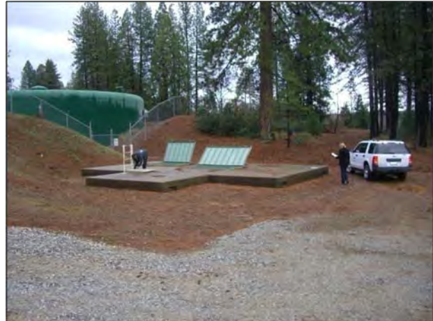
Photo 1 – El Dorado Main 2 Pressure Reducing Station No. 1 at Reservoir 3
