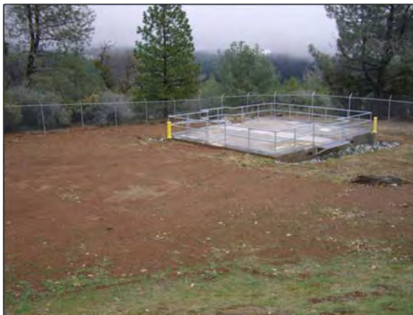
Photo 8 – Existing Pressure Reducing Station at Reservoir B
