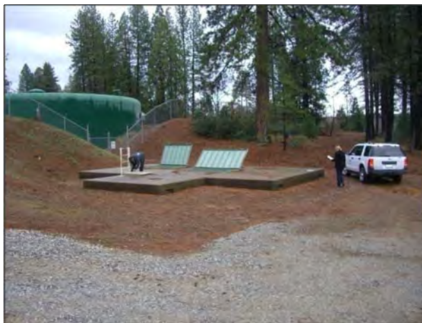
Photo 1 - El Dorado Main 2 Pressure Reducing Station No. 1 at Reservoir 3
