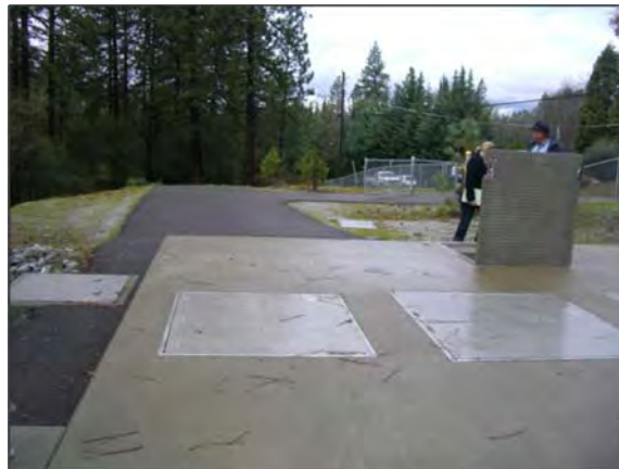
Photo 10 – DSM Pressure Reducing Station
