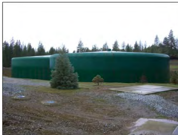
Photo 9 – Tanks and Pressure Reducing Station at Reservoir 7
