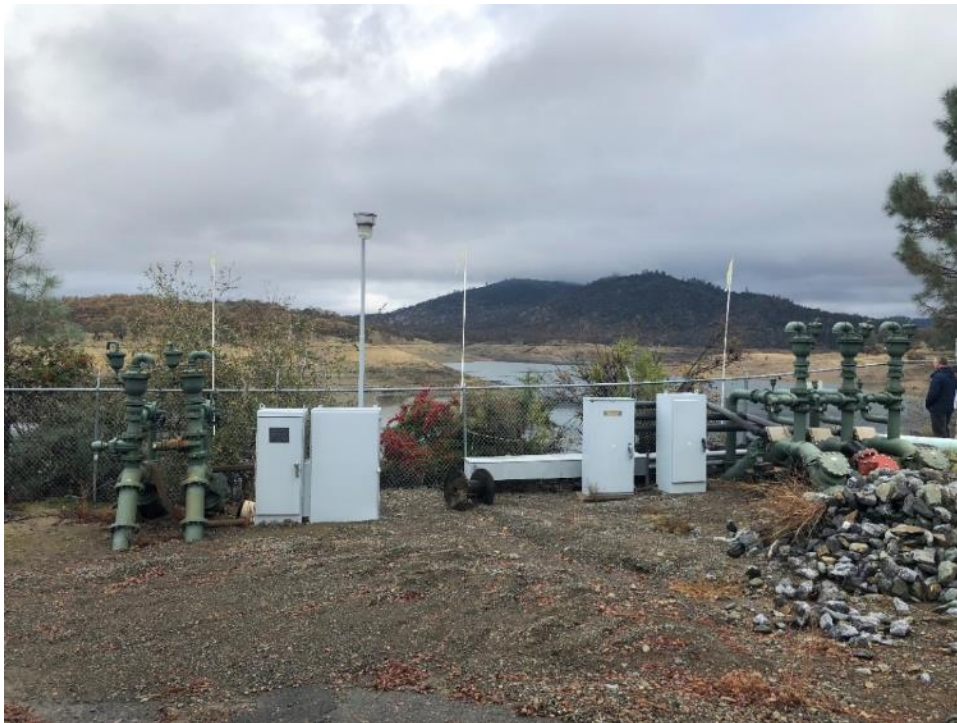
View of existing pumps to be replaced within developed portion of project site.
