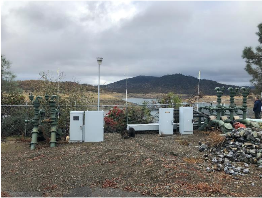
View of existing pumps to be replaced within developed portion of project site.
