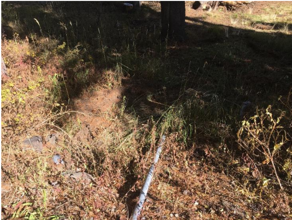
View of existing water supply line.
