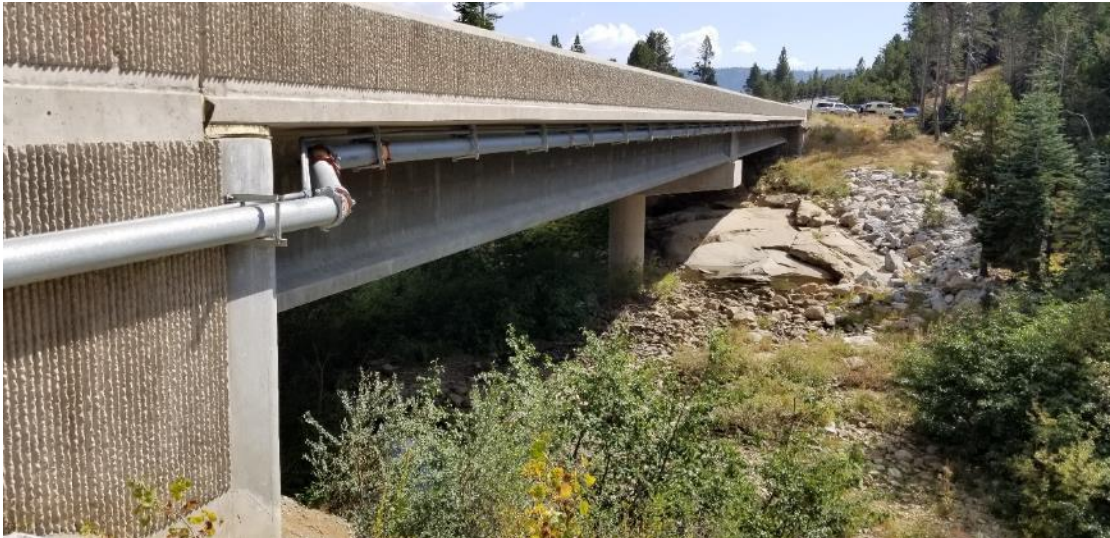
View of State Route 88 bridge where water supply pipeline will be attached, out of sight of Scenic Highway views.
