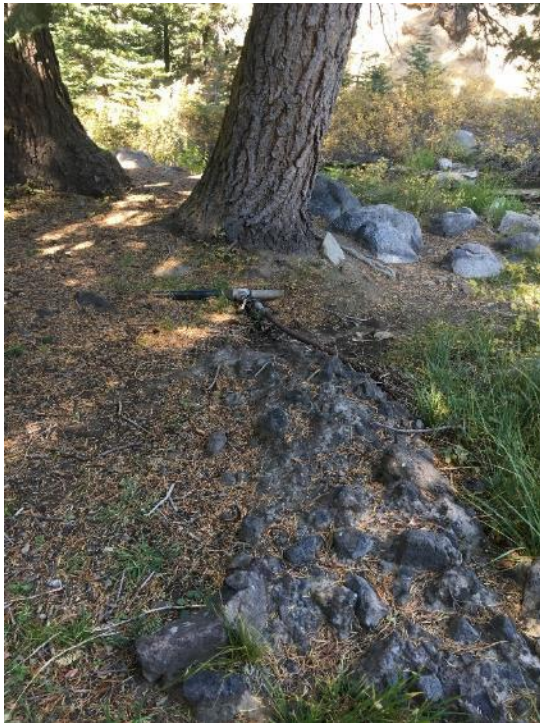
View of existing water supply line.
