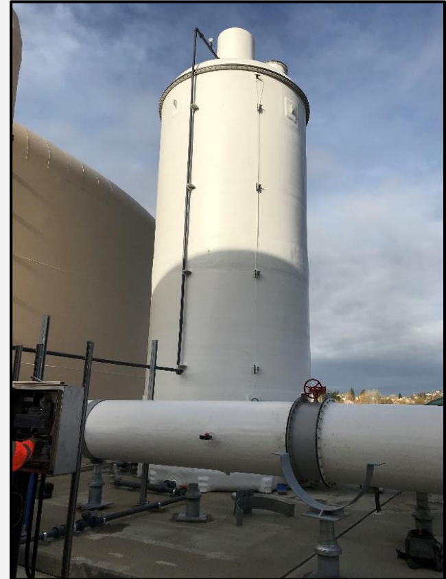
EDHWWTP Odor Control $900,000
