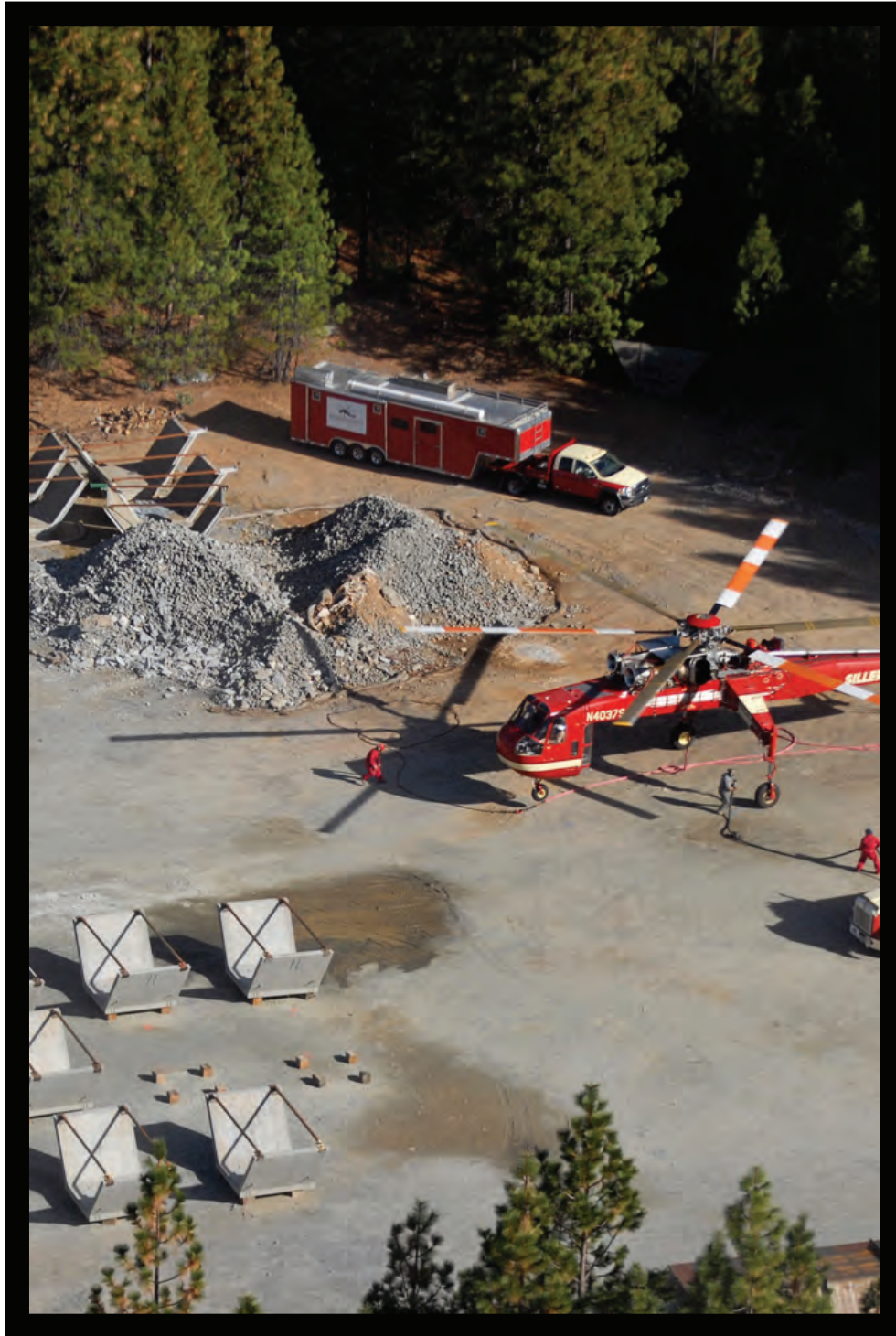
Due to the extreme terrain, a helicopter is used to place concrete sections on the Flume 9 project.
