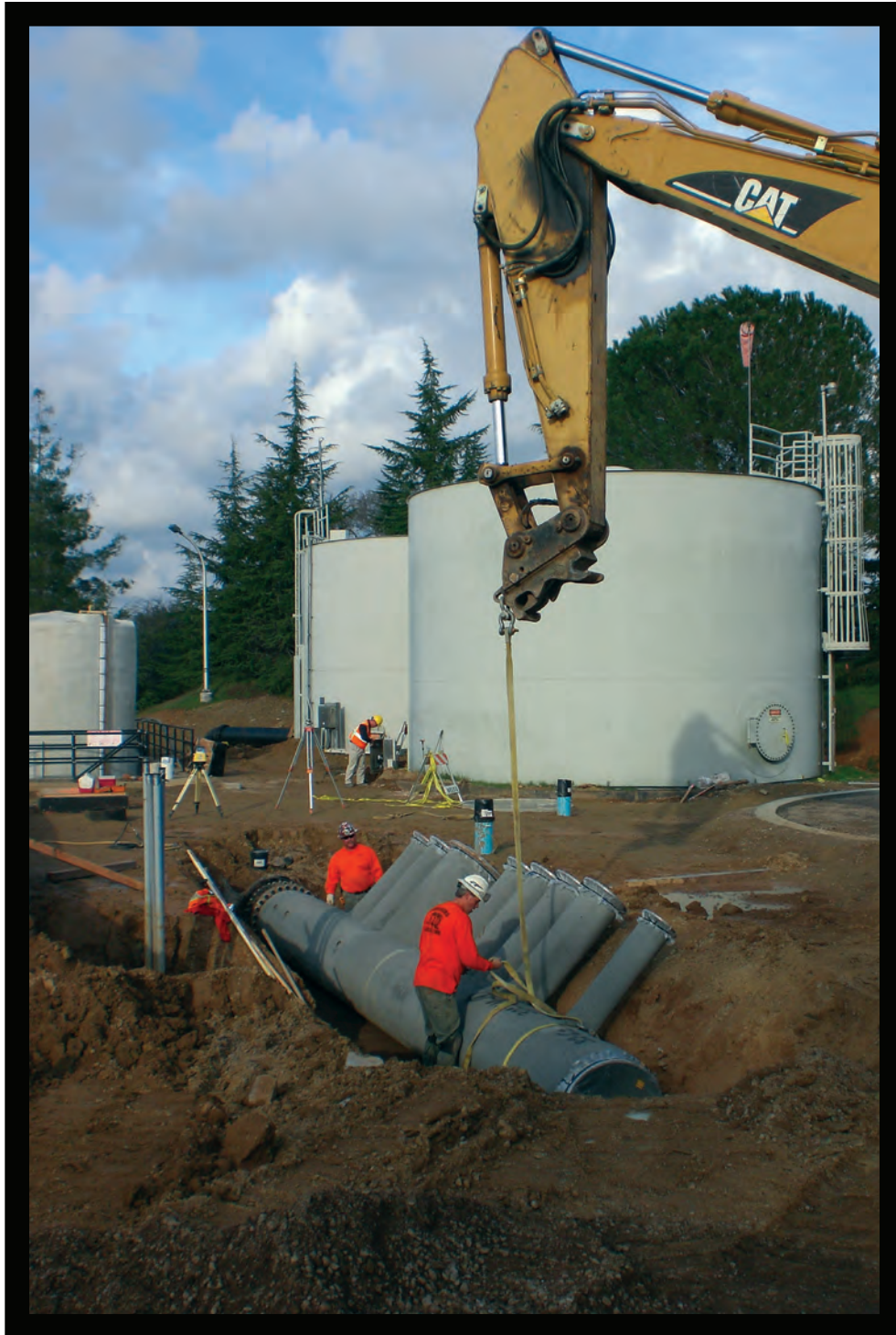
Installation of a new flash mix manifold for the $7.9 million El Dorado Hills water treatment plant expansion project.
