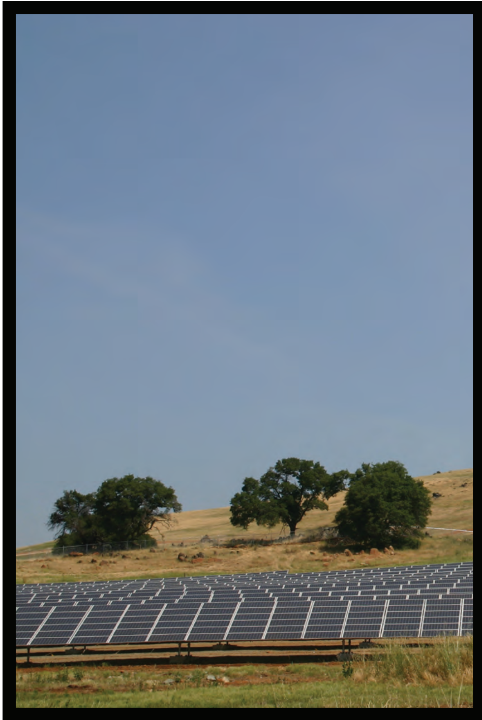
EID's 3.3 acre photovoltaic system, located at the District's El Dorado Hills wastewater treatment plant. This system, projected to pay for itself over eight years, saves several hundred thousand dollars per year in electricity bills.
