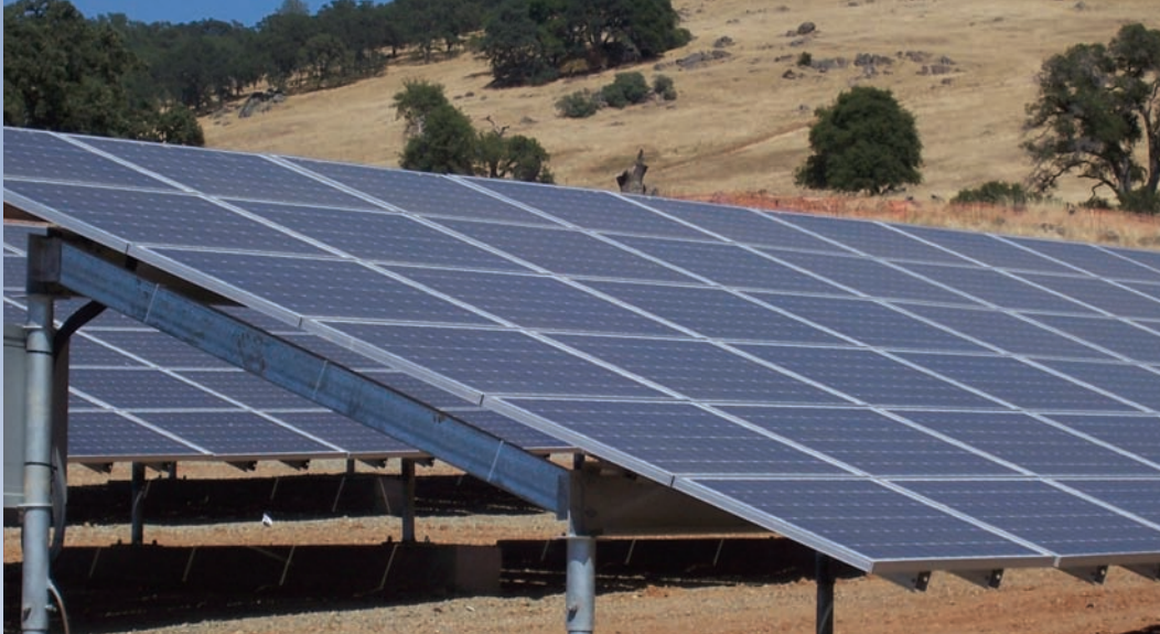
SOLAR PHOTOVOLTAIC SYSTEM AT THE EL DORADO HILLS WASTEWATER TREATMENT PLANT
