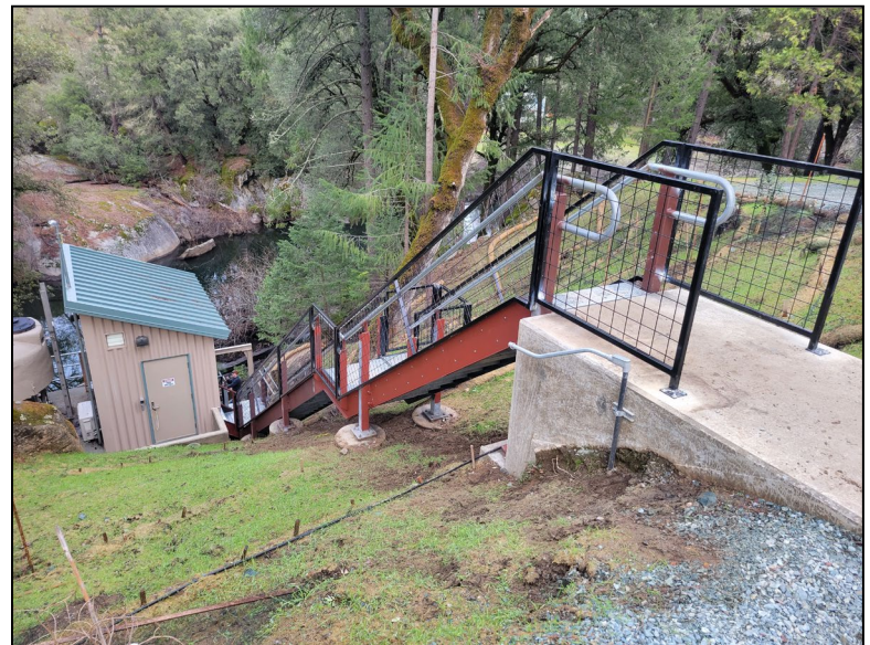
The rehabilitated dam (top), replaced intake facilities (below), and new water storage tank (not pictured) will increase the resiliency of the facilities that allow EID to serve your community
