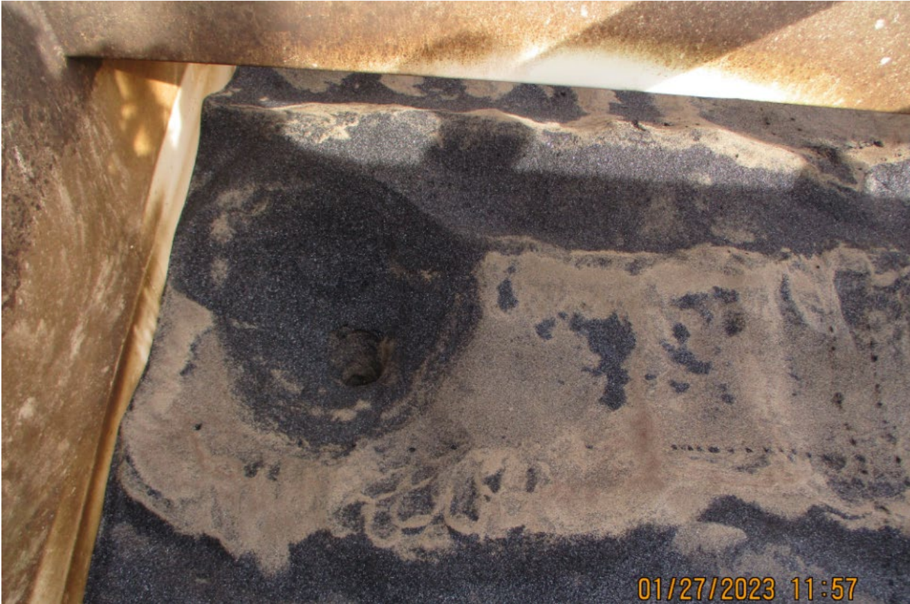
Filter 5 Multiblock Underdrain Failure
