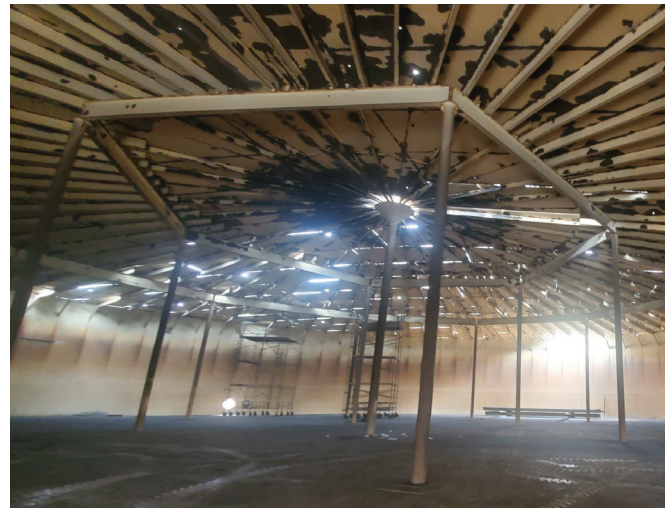
Welded steel tanks like the one shown in the pictures on this page deliver water from our eastern supplies into the El Dorado Hills area. They require regular recoating to prevent deterioration of the steel structure. The District has not been able to stay on pace with required recoating and accelerated efforts are needed to resume the required maintenance schedule. This year staff will be recoating one of the tanks on the ridge east of Bass Lake Road and next year staff are scheduled to recoat the tank within the Bridlewood community. At least one to two tanks per year need recoating to preserve these important investments.
