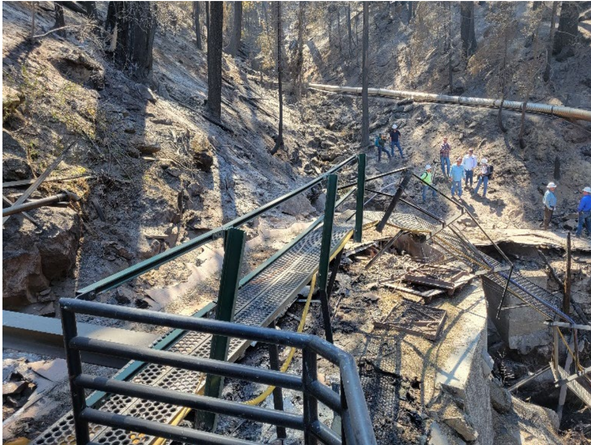
Flume 30 destroyed during the Caldor Fire.
