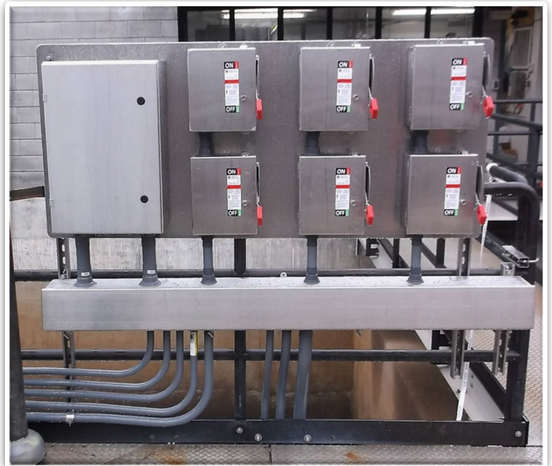
New electrical disconnects
