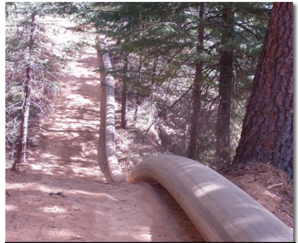
ICM inspected the CCWD Bear Creek Pipeline in very difficult mountainous terrain with high groundwater and numerous stream crossings.
