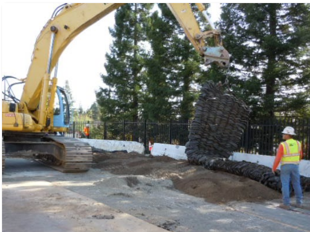
ICM provided inspection for the SJWD 72" pipeline installed in granite rock conditions. Blasting was used to excavate the trench.
