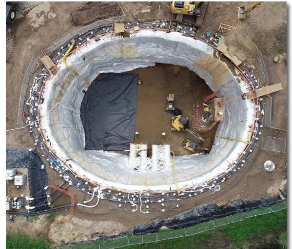
ICM provided inspection of the SRWA raw water pump station that included soil freezing to a depth of 75 feet.
