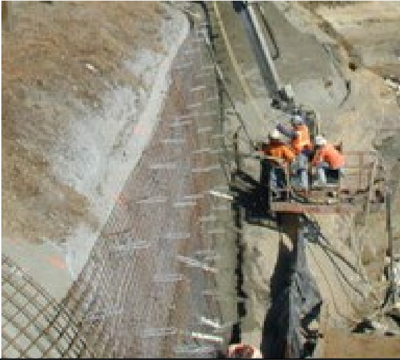
ICM inspected the Soil Stabilization Project at Red Hawk Casino (Placerville, CA)
