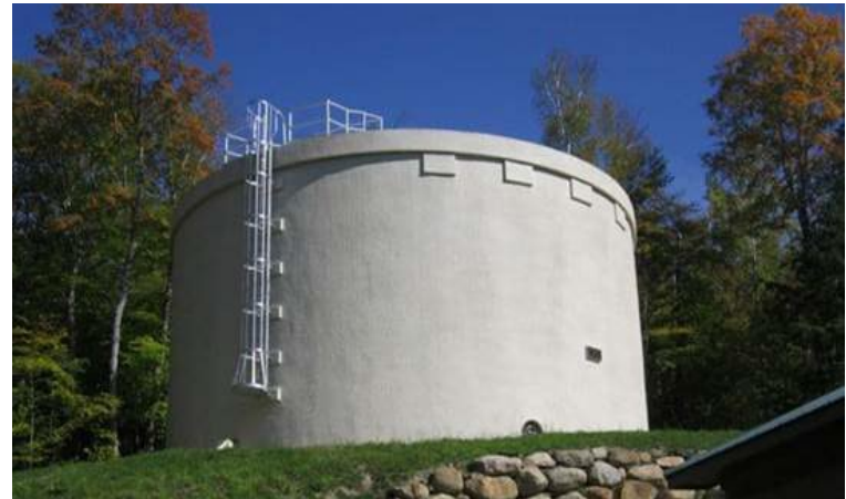
Wildfire resilient concrete tank
