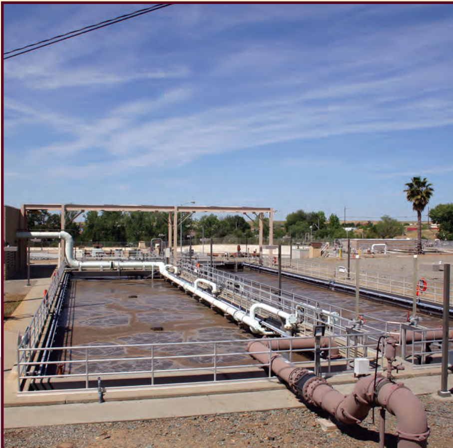
El Dorado Hills wastewater treatment plant is one of four such plants at the District.
