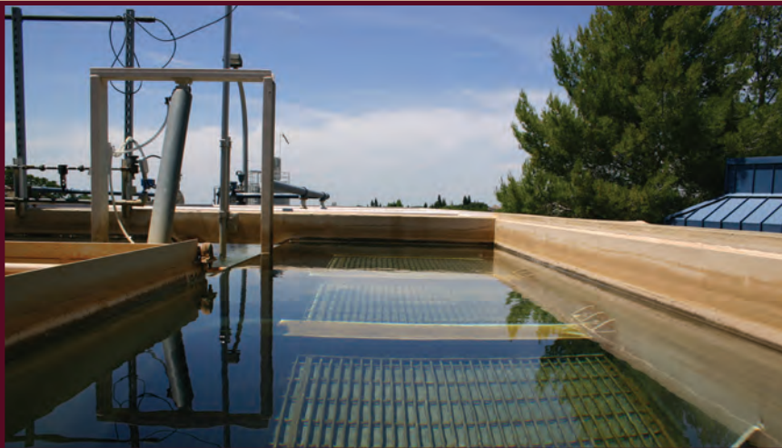
El Dorado Hills water treatment plant processed 6 million gallons of water per day when EID took over its operation in early 1973. At that time, the facility was in the middle of undeveloped land. Today, residences, a school, and a community park surround the plant. Its treatment capacity has been increased to 26 million gallons per day.
