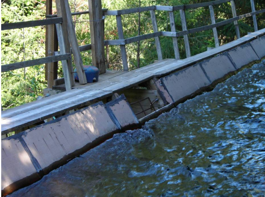
Photo A5 – Example Passive Spill
