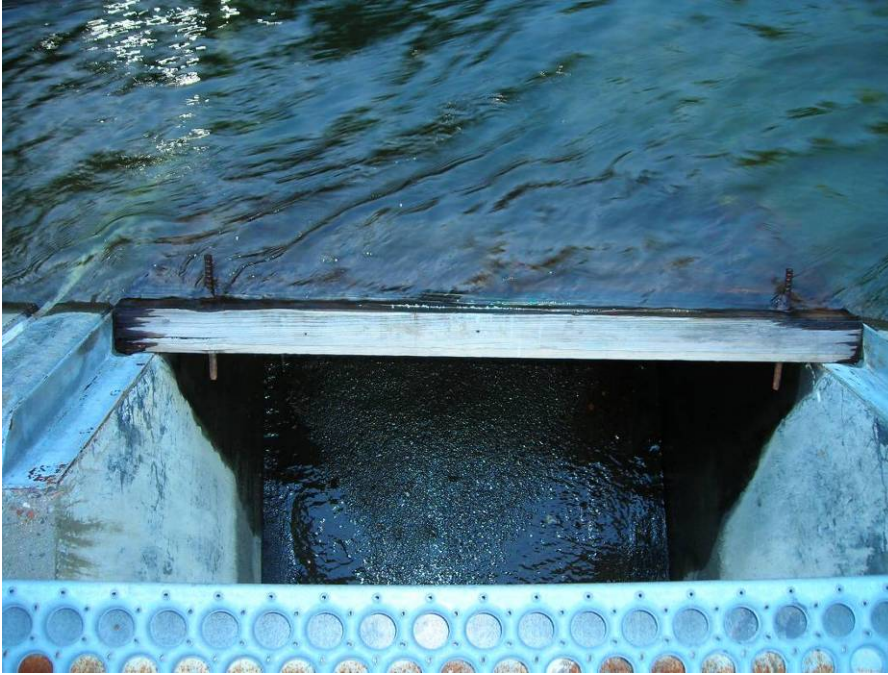
Photo A1 – Example Passive Spillway with Canal Level Controlled by Flashboards
