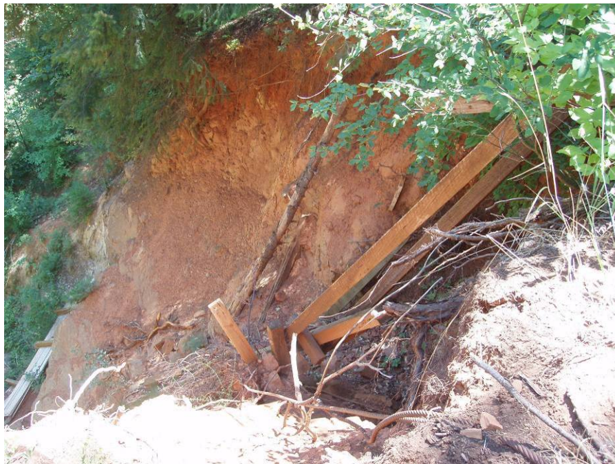
Photo B12 – Spillway 47c Headcut/Erosion
