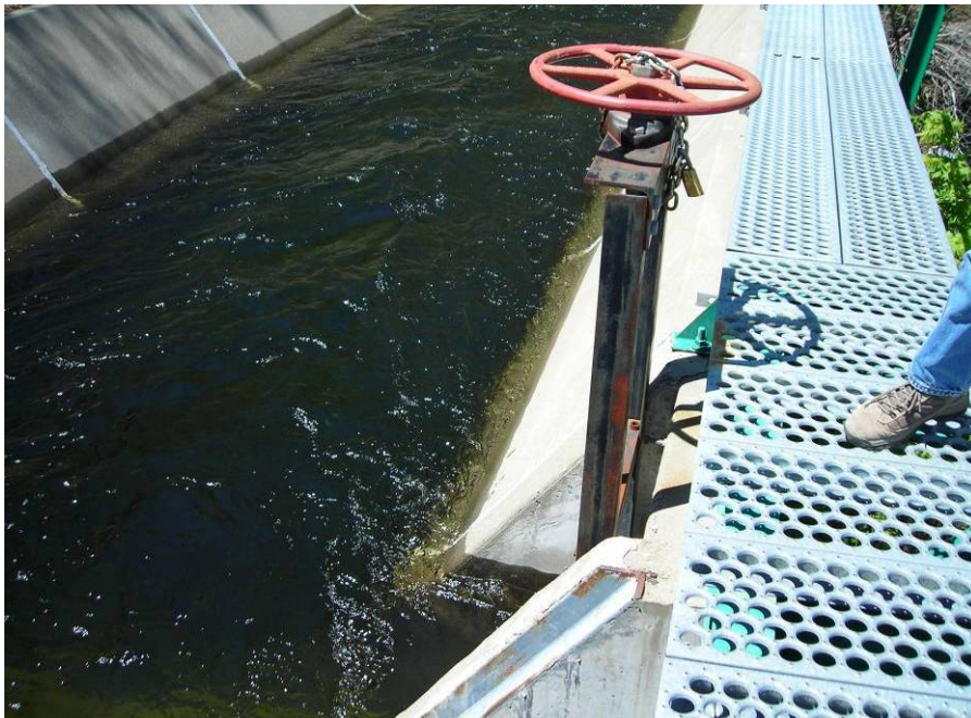
Photo A4 – Example Manual Sluice Gate with Wheel-Type Operator
