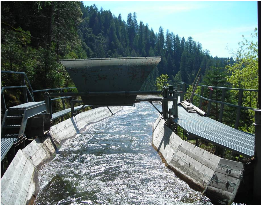
Photo A2 – Example Radial Check Gate in Open Position
