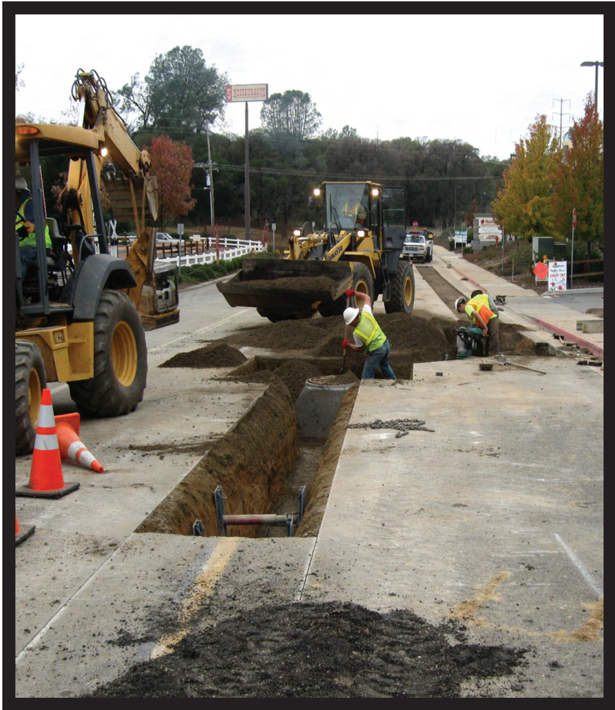
Construction crews work to replace deteriorated sewer pipe on Coach Lane in Cameron Park.
