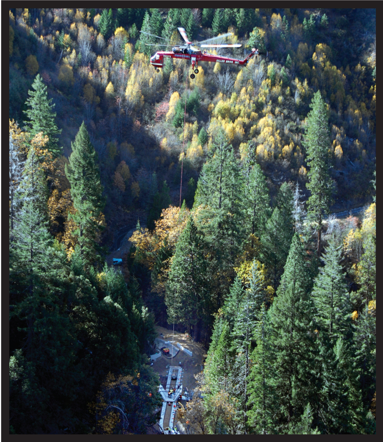
New sections of flume flown in by helicopter to replace sections of Flume 9.
