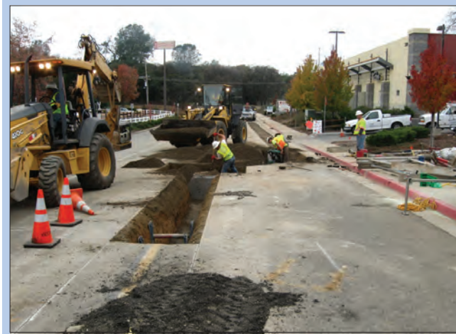
The recently completed sewer line rehabilitation along Coach Lane in Cameron Park greatly increases the reliability of the system.
