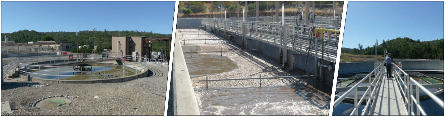
The Deer Creek wastewater treatment plant is one of four in the district. This facility treats 2.6 million gallons of flow per day.
