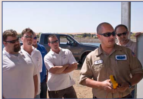
Rich Wheeler at right talks the students through the solar facility's electrical system
