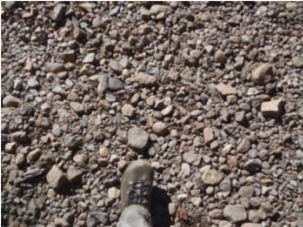
Figure A-6. Caples Spillway Channel, BI XS-3 (Lower): (a) looking upstream; (b) looking downstream; (c) looking at the left bank; (d) looking at the right bank; and (e) looking at the bed.
