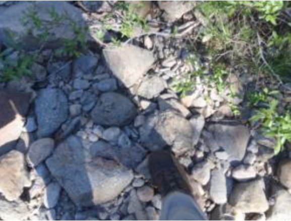
Figure A-4. Caples Spillway Channel, BI XS-1 (Upper): (a) looking upstream; (b) looking downstream; (c) looking at the left bank; (d) looking at the right bank; and (e) looking at the bed.
