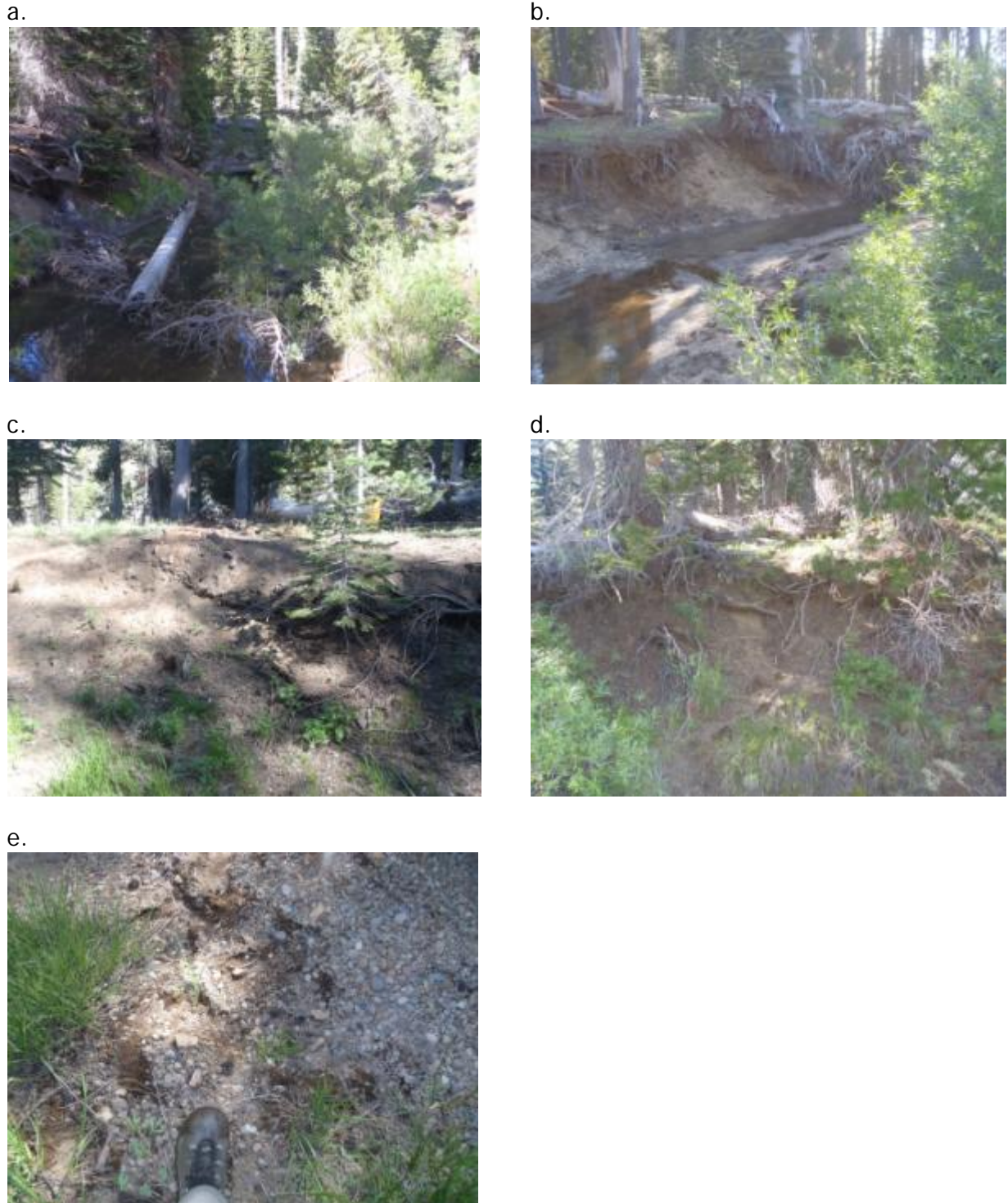
Figure A-5. Caples Spillway Channel, BI XS-2 (Mid): (a) looking upstream; (b) looking downstream; (c) looking at the left bank; (d) looking at the right bank; and (e) looking at the bed.
