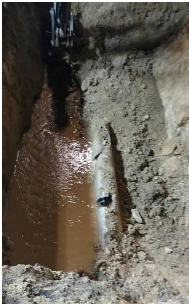
Figure 1. TCFM break at the crown of the Pipe and lateral cracking on December 16, 2016.
