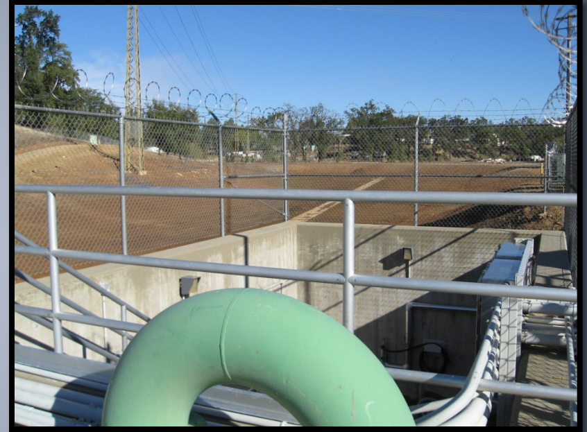
El Dorado lift station pond used to attenuate peak flows
