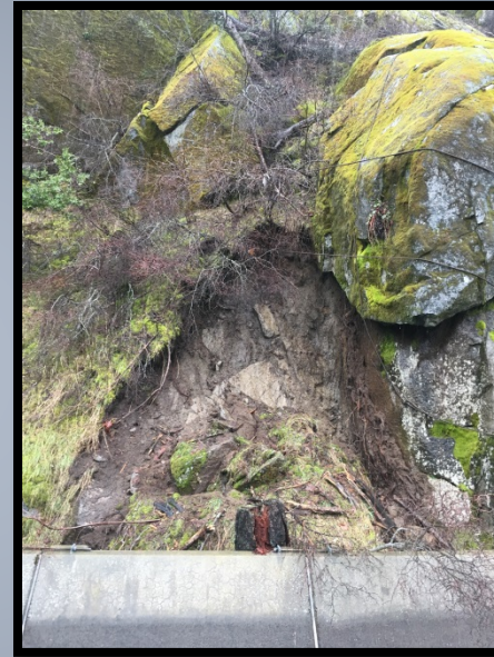
Flume 9 failure above canal 2/8/17
