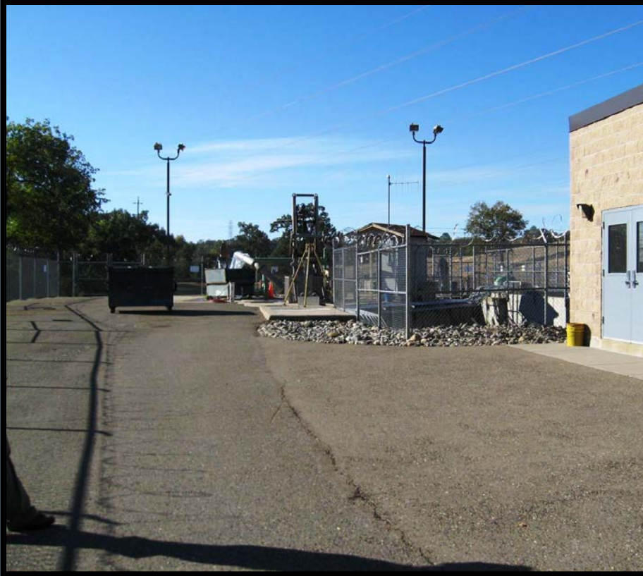
El Dorado Lift Station
