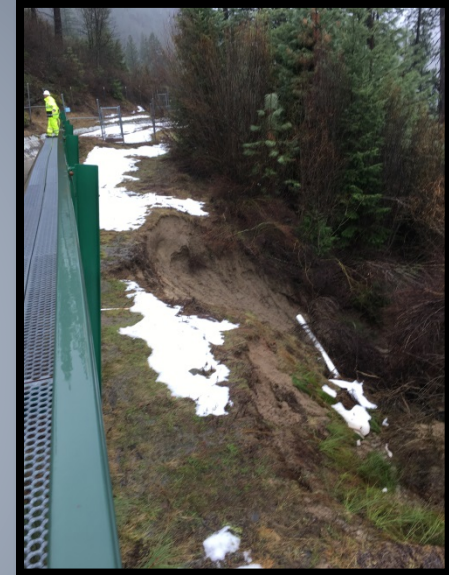
Flume 7 slide below canal 2/8/17
