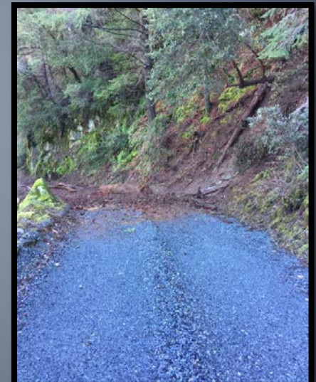
#3 Tree and debris into roadway
