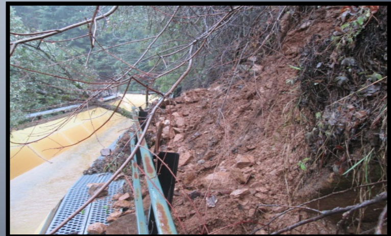
Soil impacting railing so far. Active movement anticipated until water pressure managed.
