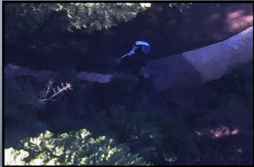
Crews creating a relief point for water blocked by material in canal
