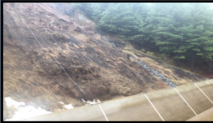
Previously installed mesh system soil movement beneath mesh
