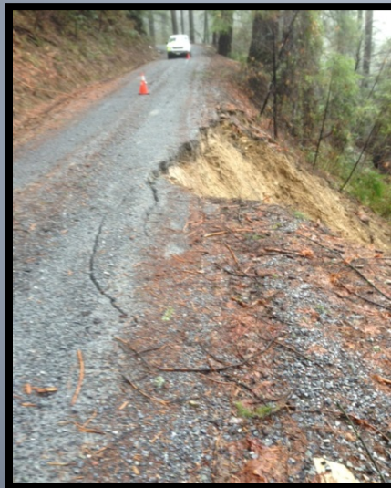
#2 Tree fell and took part of Roadway. Contractor hired.
