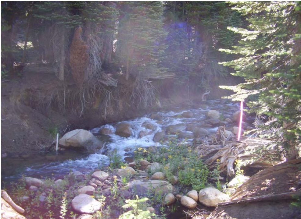
Figure 2-6 Upper Erosion Site, view upstream of right bank (left bank also eroding, not in view)
