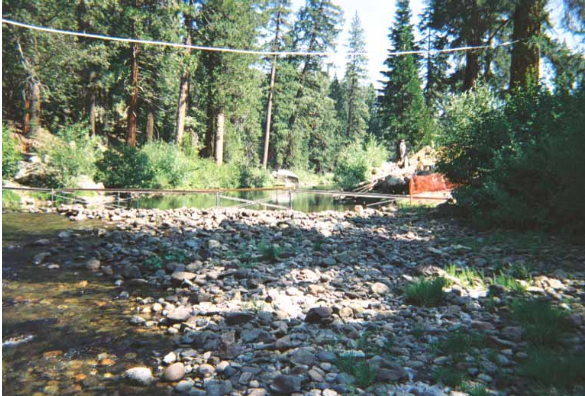
Figure 31: Silver Fork at China Flat (site #16), upstream view of bridge replacement construction, August 2002
