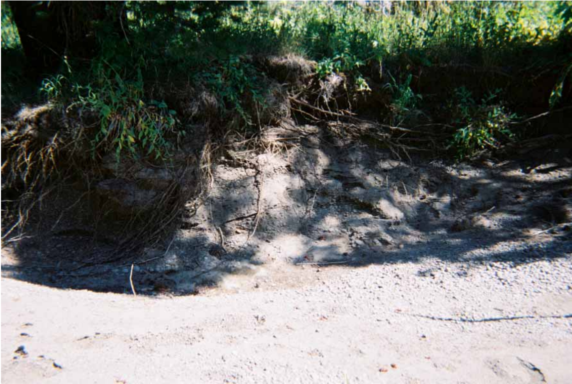
Figure 40: Lost Axe, unnamed tributary of Caples Creek (site #13), cross -section view of right bank, August 2002
